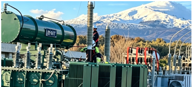
Italy | Enel 150kV Natural Ester Transformer
