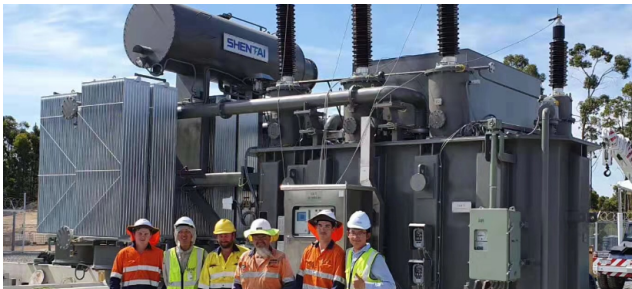
Australia | 132kV Natural Ester Transformer
